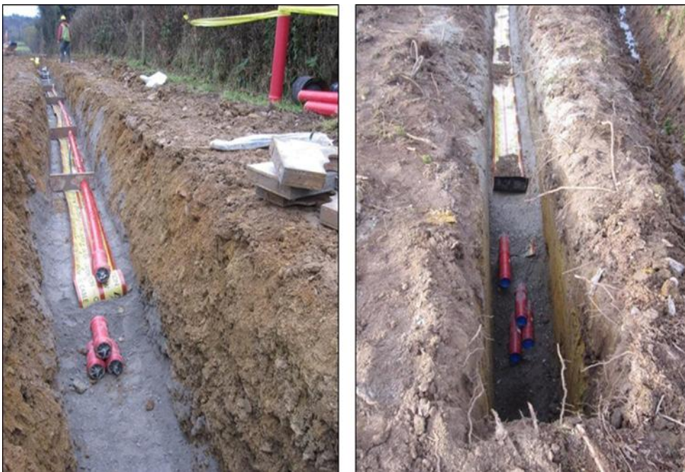
Plate 2-2 Typical Trefoil Cable Trench View
